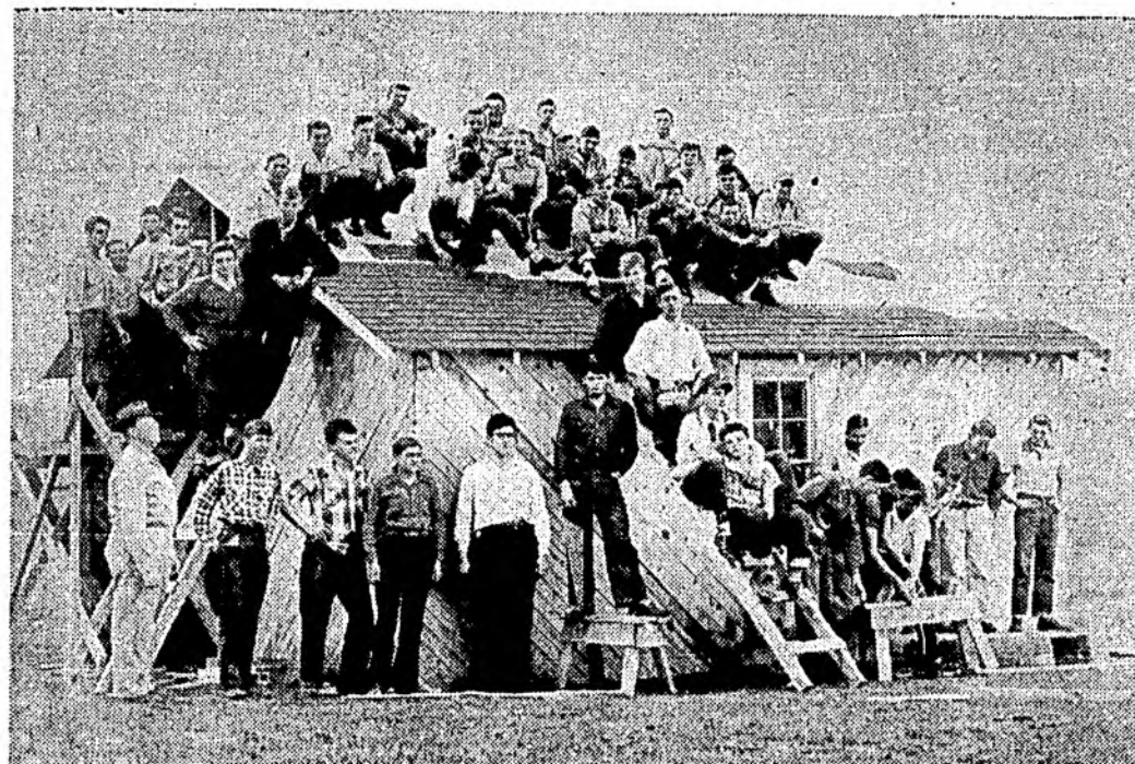
"LEARNING TO DO BY DOING"—The agricultural classes of the Farmington High School are currently engaged in the construction of a garage-storage building on a farm near the school. Forty-six boys are engaged on this project, under the direction and supervision of J. E. Sherill, Vocational Agriculture Teacher. (Enterprise Photo).
